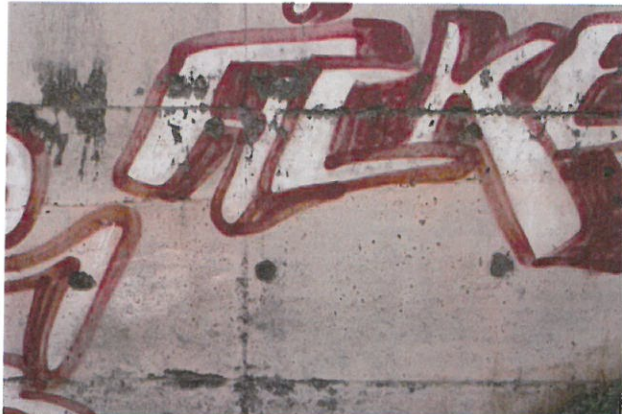
RISSE WIDERLAGER WEST
